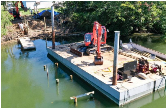
The pier on Pitmans Cove, off Indian Creek, at Camp Kekoka, Kilmarnock, Virginia, under construction
